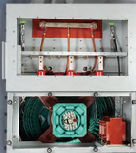
High Voltage with Rear Cover Removed
