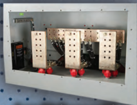
Low Voltage with Rear Cover Removed
